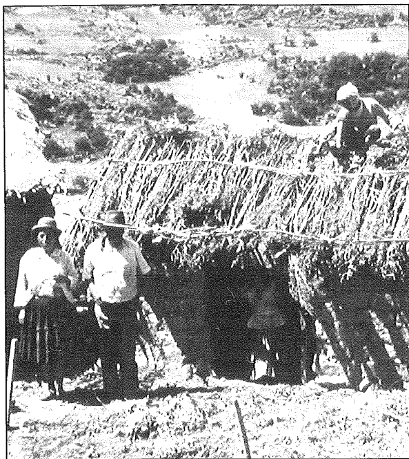
B. A roof is constructed using branches of kewina ( Polylepis besser ) covered with thola ( Baccaris obtusifolia ).
